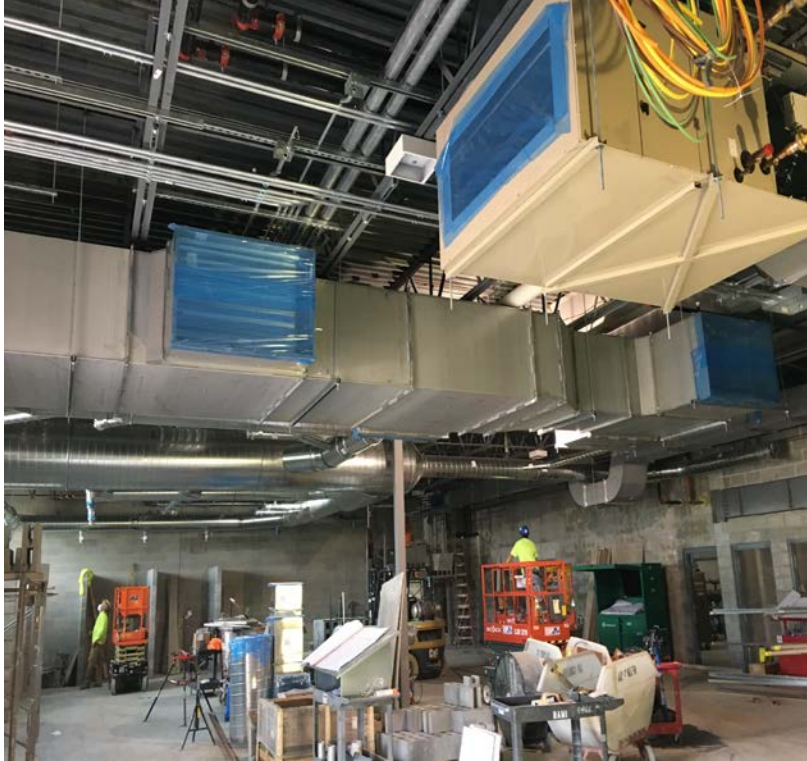
Tech Ed mechanical installations
